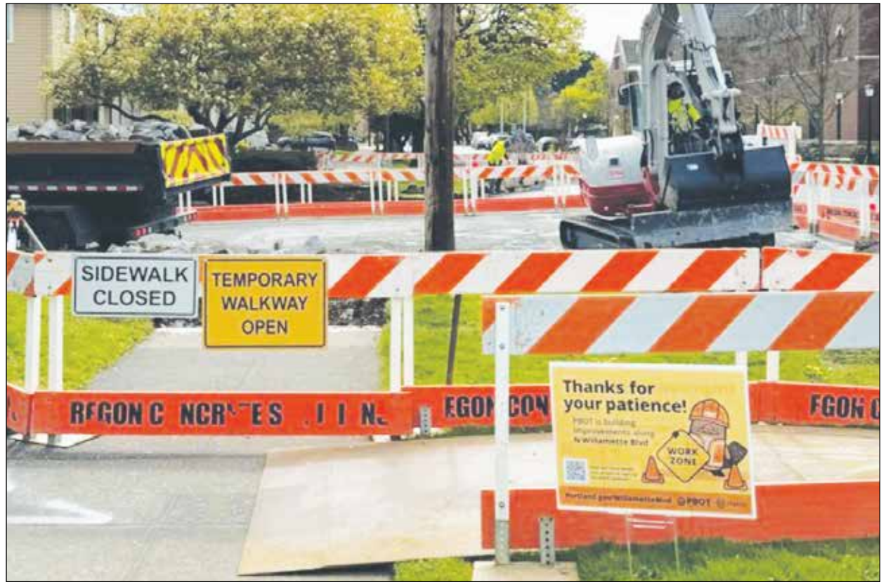
Portland Transportation Bureau crews work on a corner of North Willamette Boulevard. Paving is starting this month. (PBOT)
