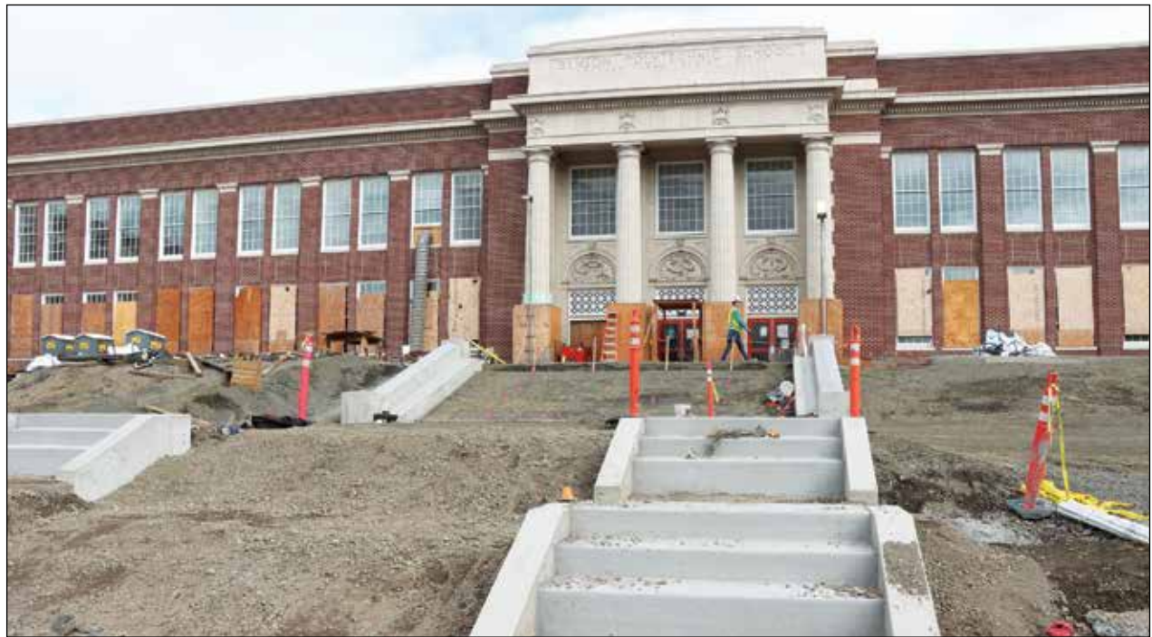
These photos show the work that is continuing at Benson High School where a modernization project is scheduled to be completed in the summer. Several weeks ago, terracotta details on the main building's exterior were cleaned and repaired, and the original windows were rehabilitated and reinstalled. (Portland Public Schools)
