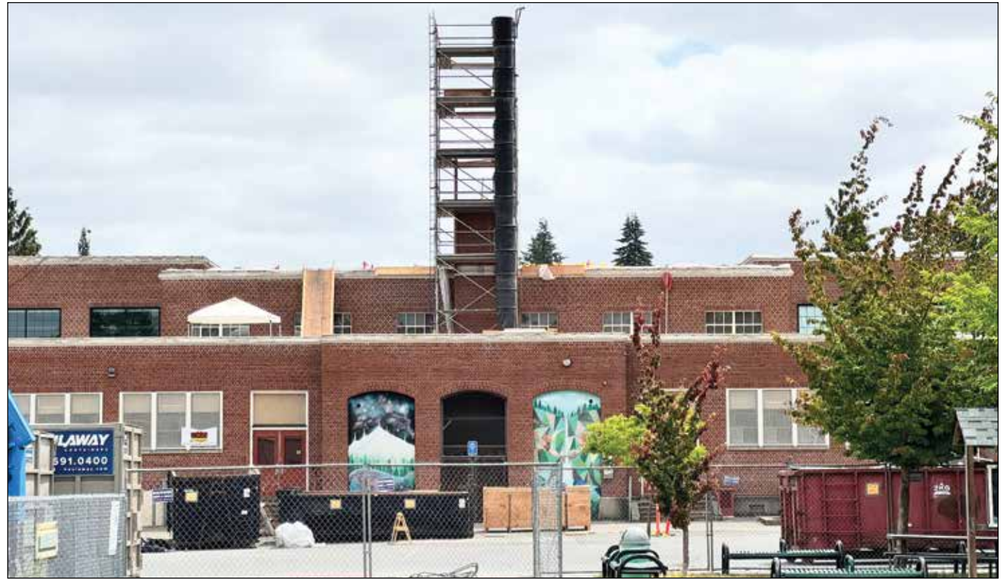
Crews removed a century-old brick boiler chimney from Vestal Elementary School in Montavilla. The work is part of a larger update for the century-old building that will include a new roof, new skylights and updated gym windows. (Jacob Loeb/Montavilla News)
