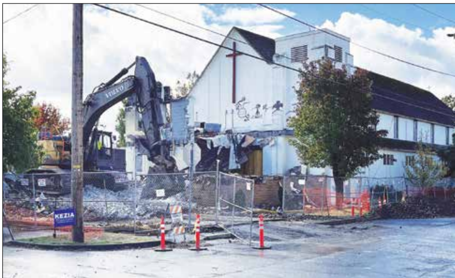
The Word and Spirit Church in Rose City Park was damaged in a January fire and is being deconstructed to make way for 20 new living units. (Phill Colombo)
