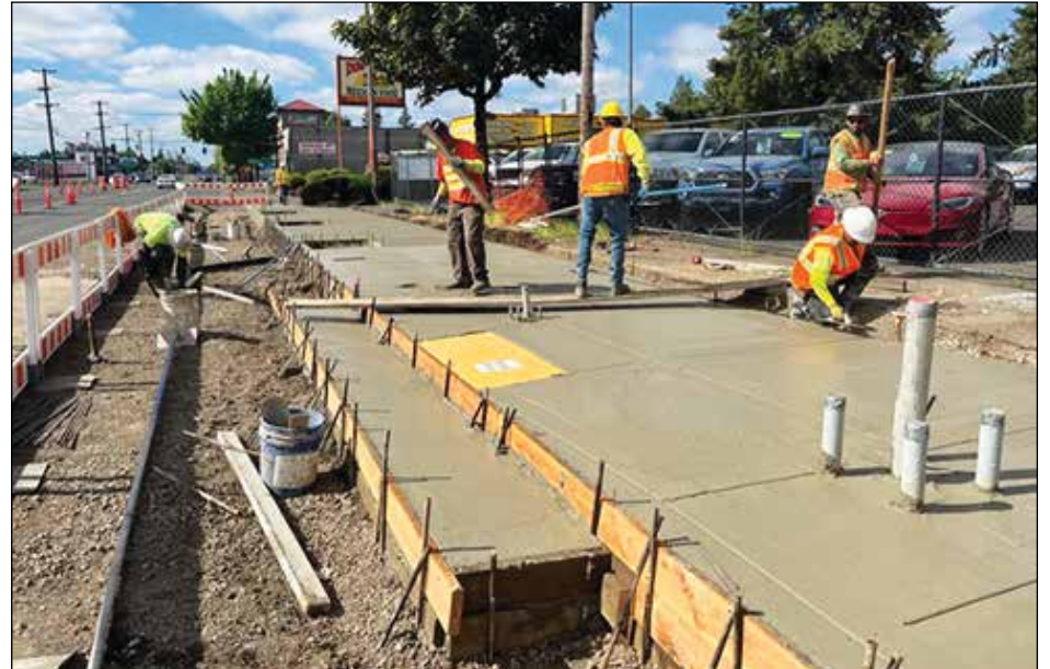
Construction crews finish concrete for an ADA corner ramp at Southeast 82nd Avenue and Schiller Street, one of the many projects Portland’s Bureau of Transportation has started work on since taking ownership of 82nd Avenue in 2022. (PBOT)
